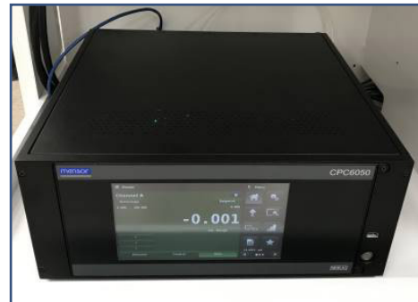
Mensor pressure controller installed in internal instrument bay.
